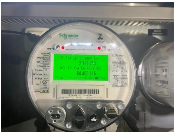
Meter 3 (UTE 2 – Central Energética Tupaciguara - Main)
