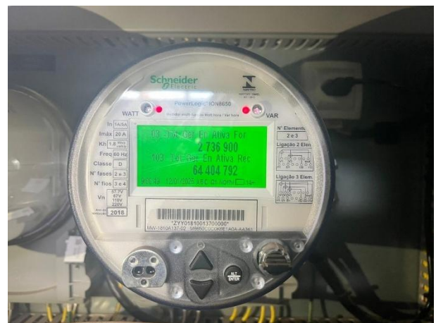
Meter 4 (UTE 2 – Central Energética Tupaciguara - Check)
